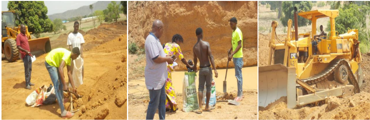
Fig.11: Samples collection at Dabi site where Dantata and Sawoe Construction Company is using for Gwagwalada-Kwali road construction.
