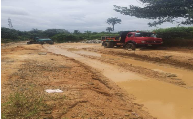
Plate 2: Heavily damaged roads at Choba mining site.
