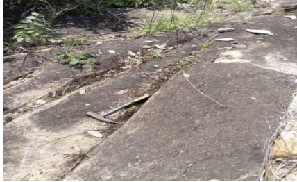
Plate 9: Fractures present in granite
