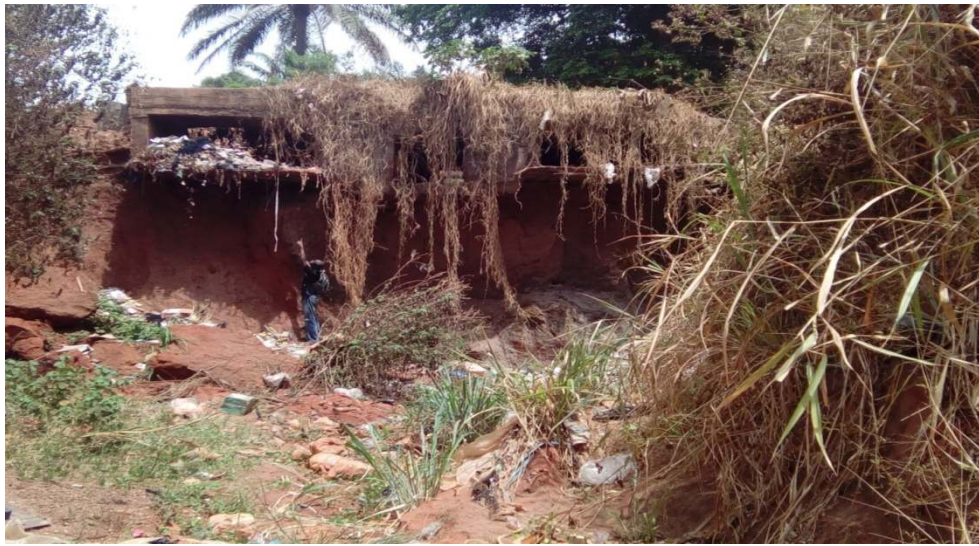
Plate E: Gully erosion at Onuiyi Road Culvert in 2016 (Note the author, whose height is almost half way the gully depth at 1.9 m)
