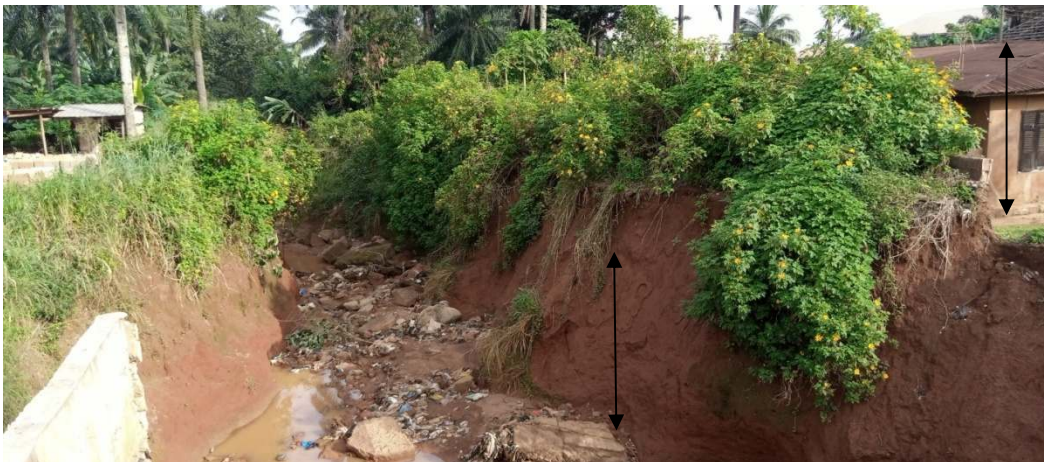
Plate F: The same gully erosion at Onuiyi Road Culvert in 2020 (Note the house around the gully site, with the height of the house about half of the gully depth at 3.84 m)
