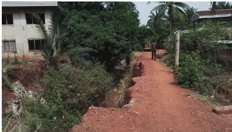
Plate H: Gully cut at Ibeziako Street with the street reduced to a footpath and house endangered by the gully in 2016
