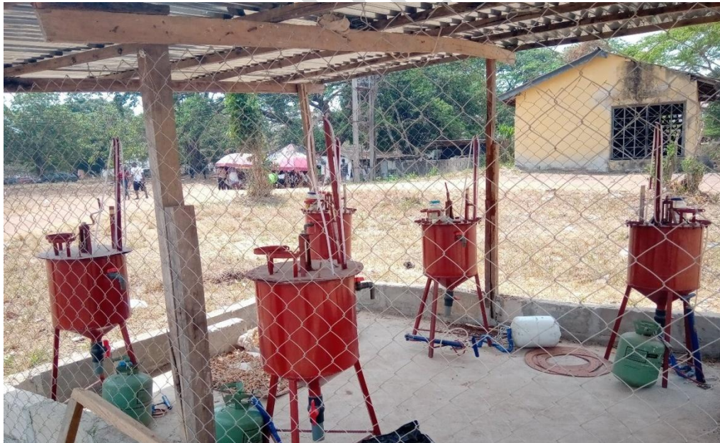
Plate 1: Locally fabricated biodigesters
