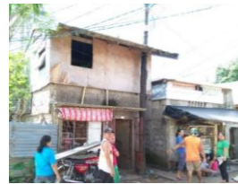
Poor building design
