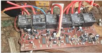
Fig. 2. The Charge Controller
