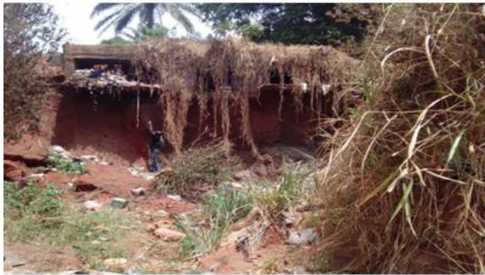
Plate E: Gully erosion at Onuiyi Road Culvert in 2016 (Note the author, whose height is almost half way the gully depth at 1.9 m)
