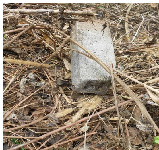
Photo 4: Pillar displaced by unsatisfied 15
