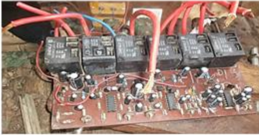
Fig. 2. The Charge Controller
