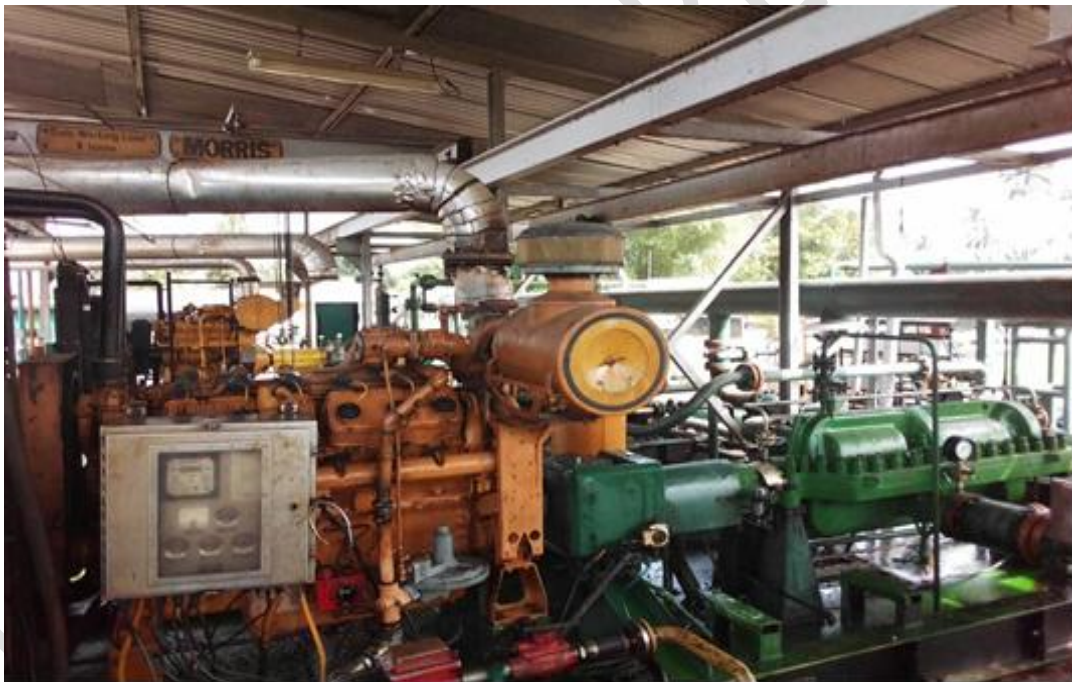
Plate 1 GAS LIFT COMPRESSOR Source: Author's field work, 2020
