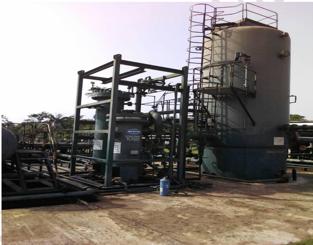
Plate 2 SURGE VESSEL Source: Author's field work, 2020
