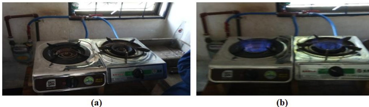
Fig.8. (a) Installed biogas stoves that are turned off when not in use. (b) Installed biogas stoves that are turned on when in use.
