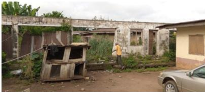
Plate L: The same property completely destroyed by the gully in 2020
