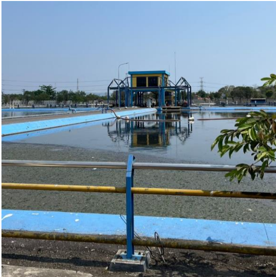
Figure 1. Sewon WWTP in October 2023
