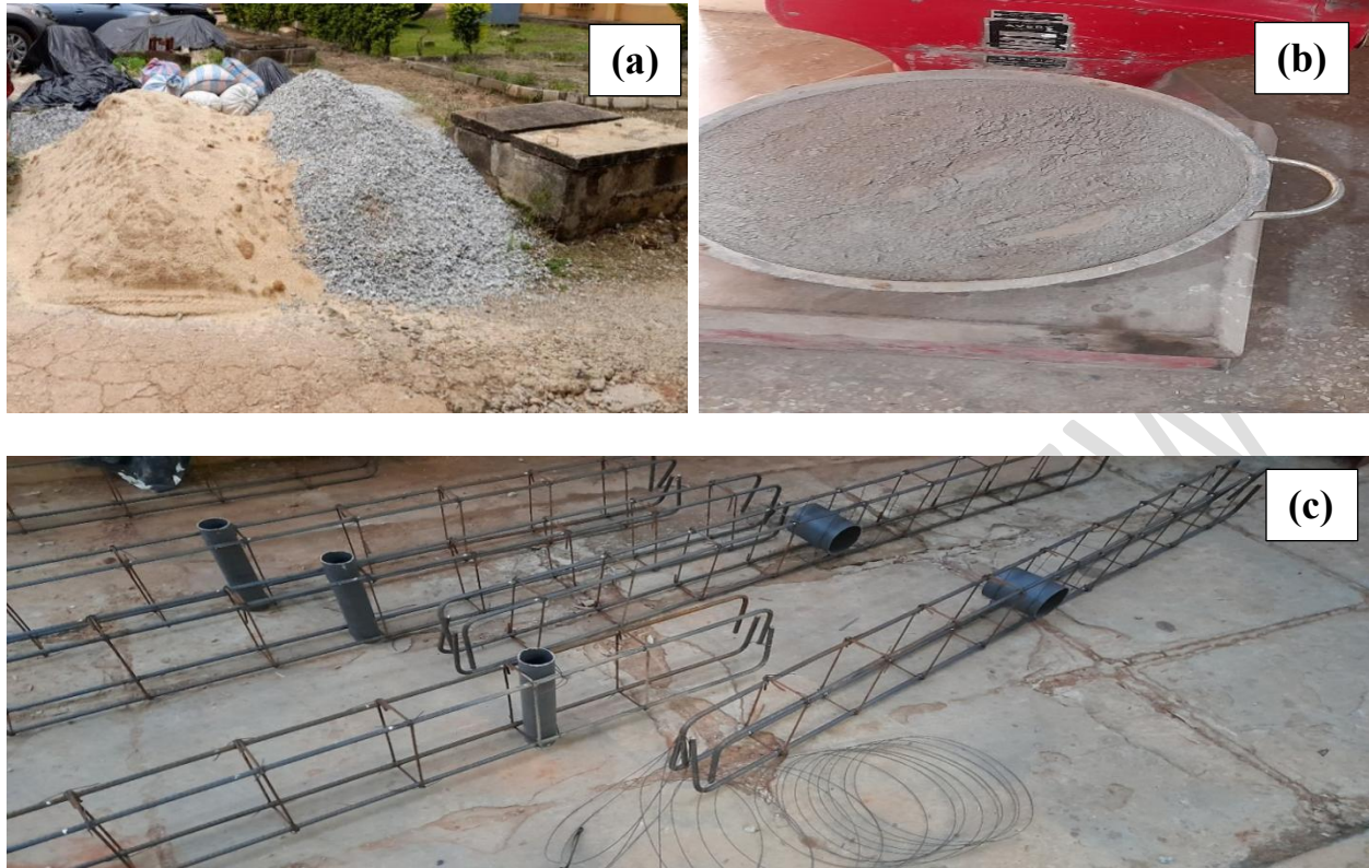
Fig. 1. Materials: (a) sand and gravel, (b) cement, (c) 12mm steel rebars with 8mm stirrups and PVC pipes.
