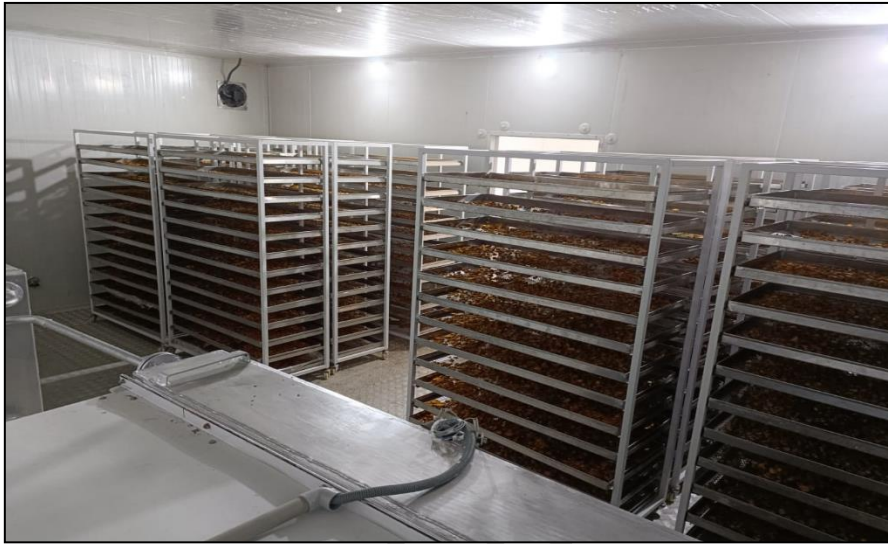
Plate 1 Full load testing of drying system
