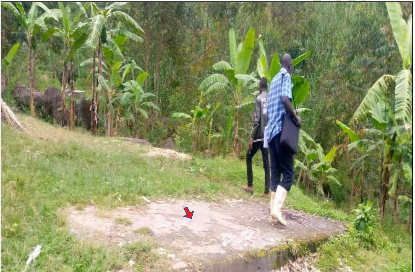
Figure 2: Representative images of the remains of Nametsi Health Center II (Red Arrow), that was sunk by landslides in Bududa District, Eastern Uganda
