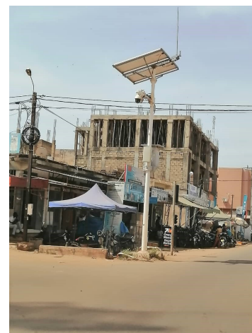
Figure 1: Surveillance camera powered by PV energy to control road traffic in the City of Ouagadougou (Burkina Faso)
