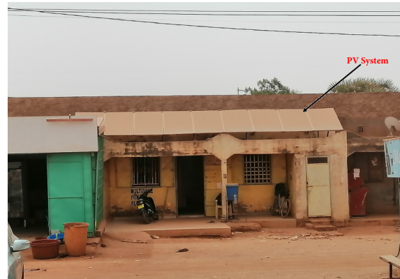
Figure 3: PV system in roofing of shop in Ouagadougou City
