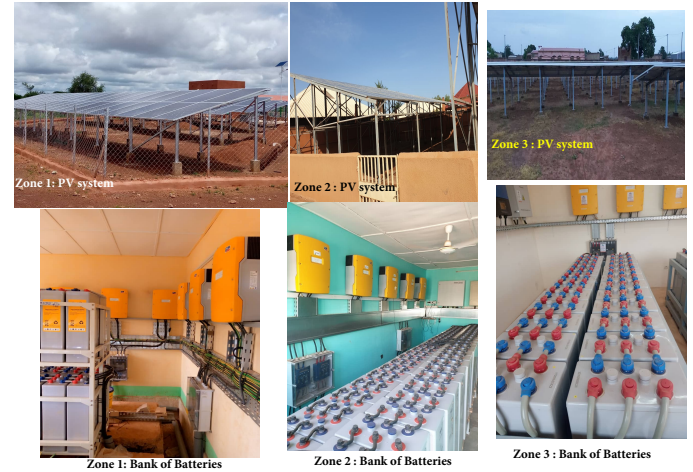
Figure 6: 50kW_p power plant installed in the three climatic zones of Burkina Faso
