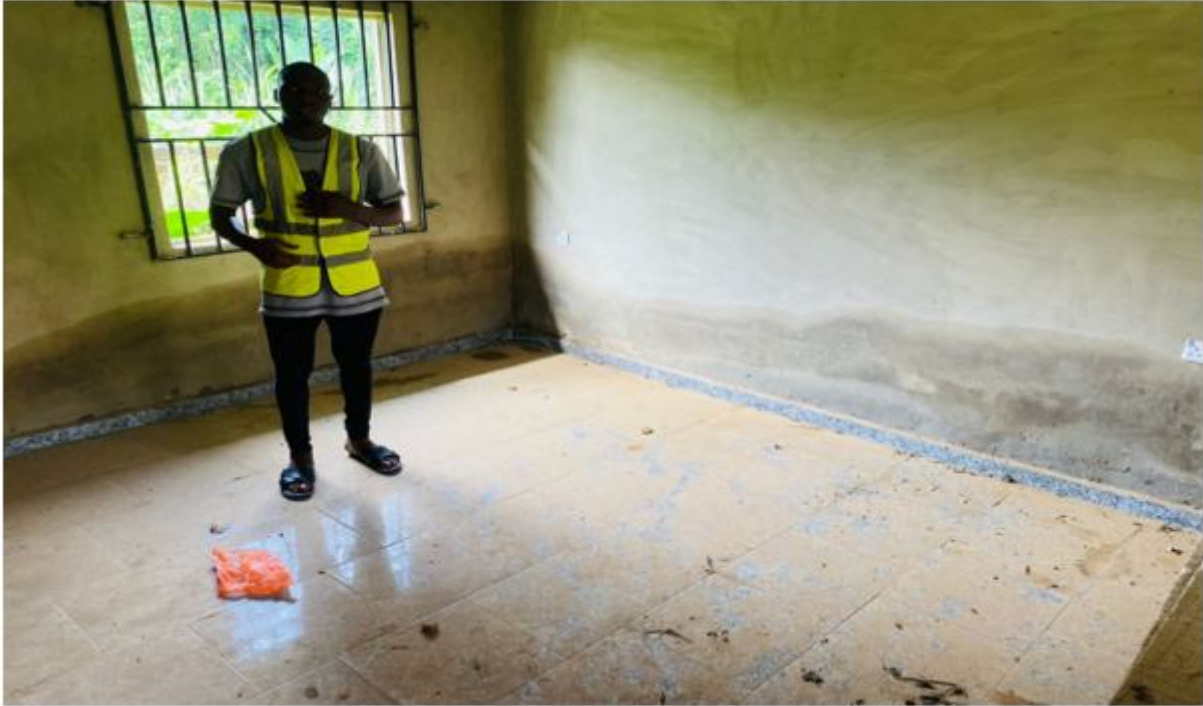
Plate 6: A building with damp, which leads to functional failures
