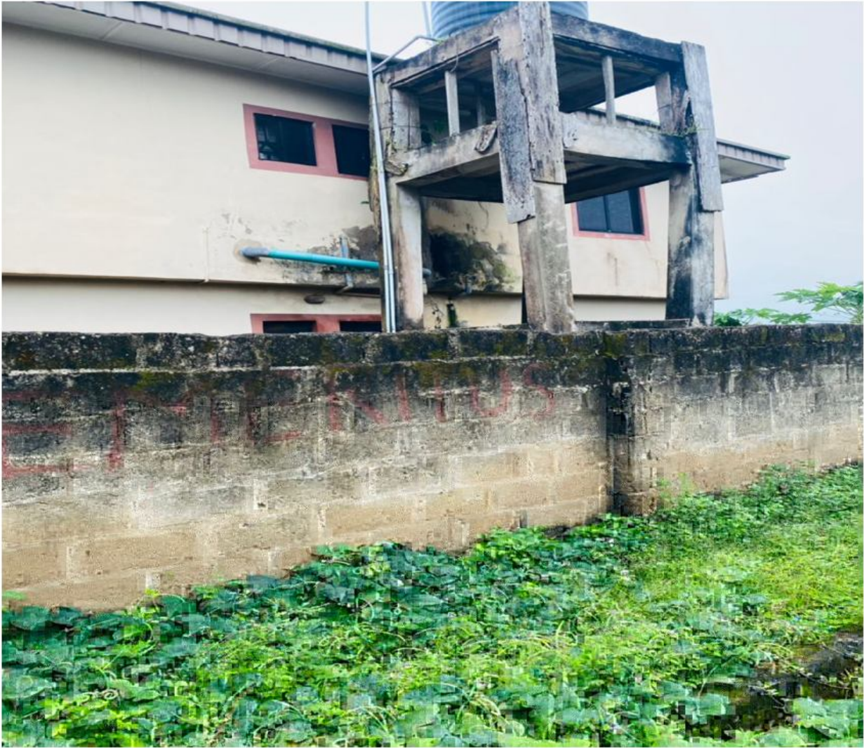
Plate 9: Buildings with plumbing defect
