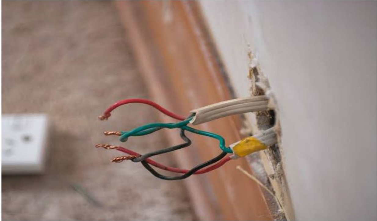
Plate 5: A building with electrical wiring defects which leads to functional failure.
