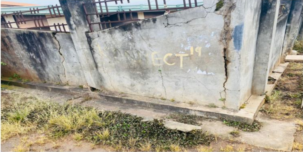
Plate 8: Buildings with cracks
