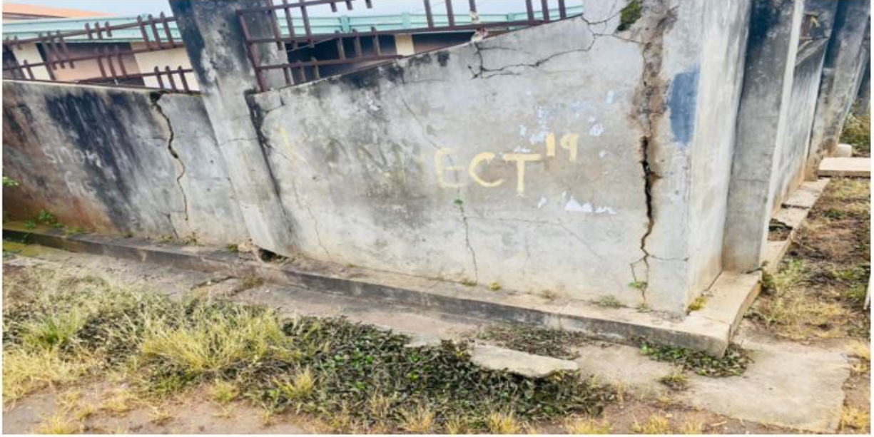
Plate 8: Buildings with cracks
