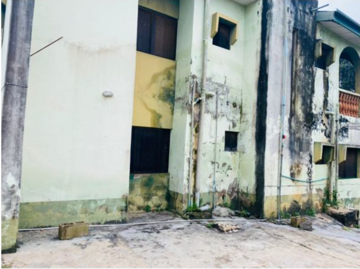
Plate .1: Buildings with functional failure as a result of damp
