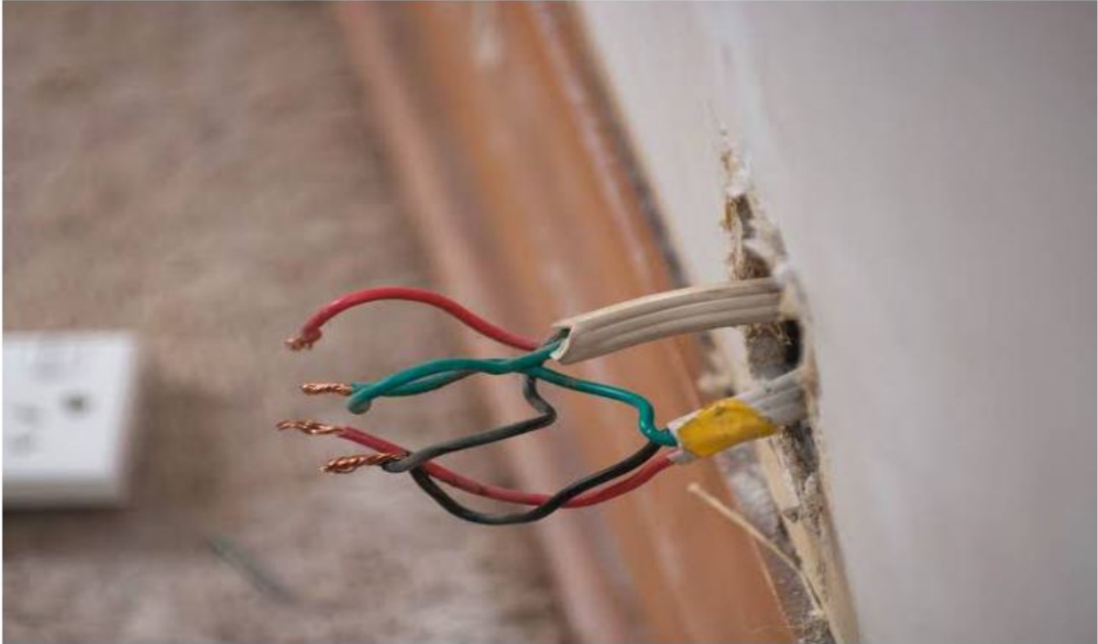
Plate .5: A building with electrical wiring defects which leads to functional failure.
