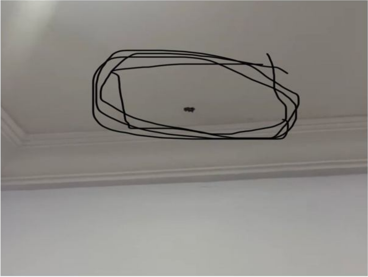
Plate .2: Roof defect.
