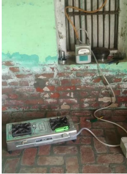
Fig.3: Installed Biogas flowmeter at village Dholu Plant
