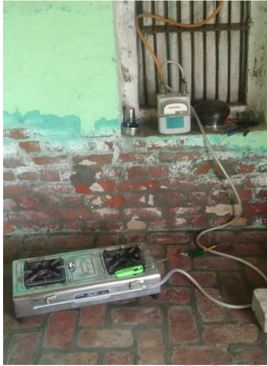
Fig.3: Installed Biogas flowmeter at village Dholu Plant
