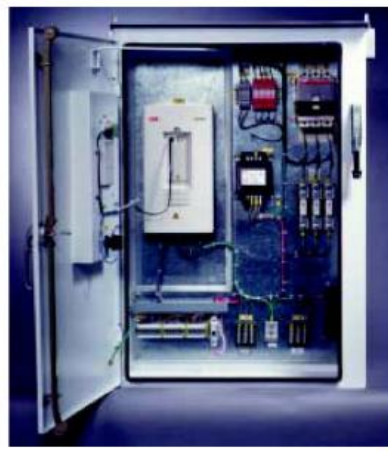
Figure 5. ABB ALC 600 controller
