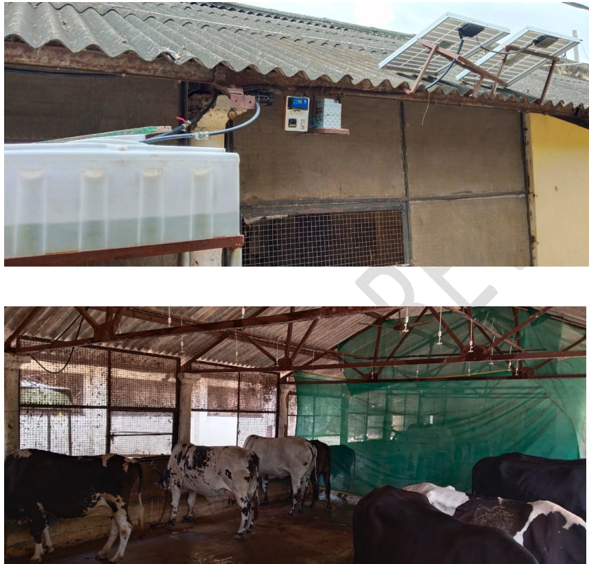
Fig 8. Solar powered cooling system in a cattle housing structure
