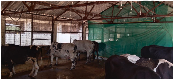
Fig 8. Solar power-assisted cooling system in an animal housing structure
