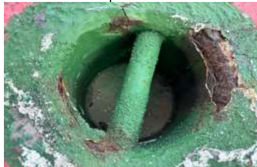
Fig. 4. Helideck surface degradation around the tie-down points
