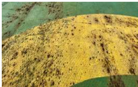
Fig. 5. Degradation of helideck surface around the Touchdown and position marking circle leading to reduced surface friction
