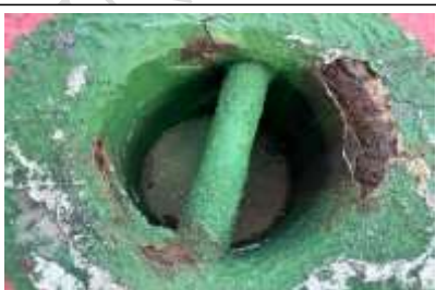
Figure 5: helideck surface degradation around the tie-down points.
