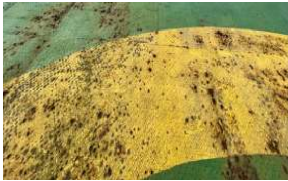
Figure 6: Degradation of helideck surface around the Touchdown and position marking circle leading to reduced surface friction.
