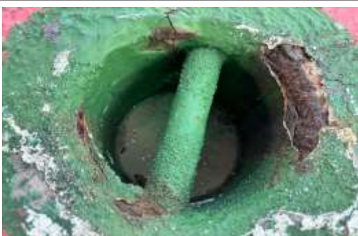
Figure 5: helideck surface degradation around the tie-down points.
