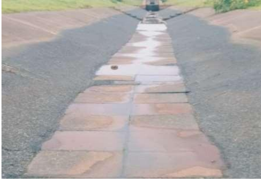
Figure 4: Differential Movements on the Precast Concrete
