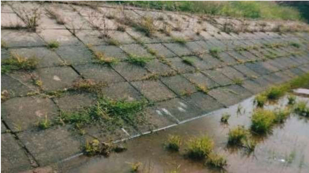
Figure 6: Vegetation and Grass Growth on the Joints of Precast Concrete
