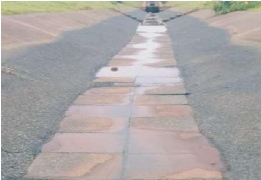
Figure 4: Differential Movements on the Precast Concrete
