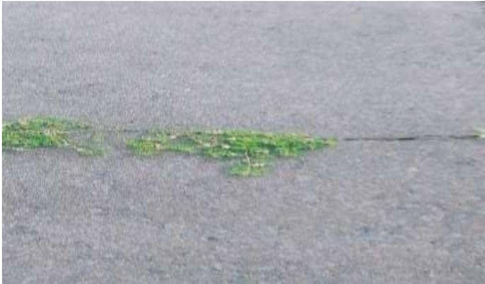
Figure 7: Vegetation and Grass Growth in the Cracks of Insitu Concrete
