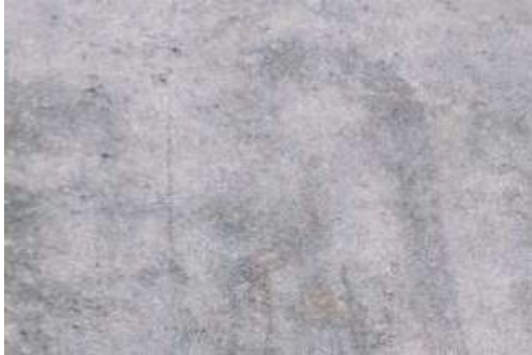
Figure 5: Effect of Rainfall on the Insitu Concrete
