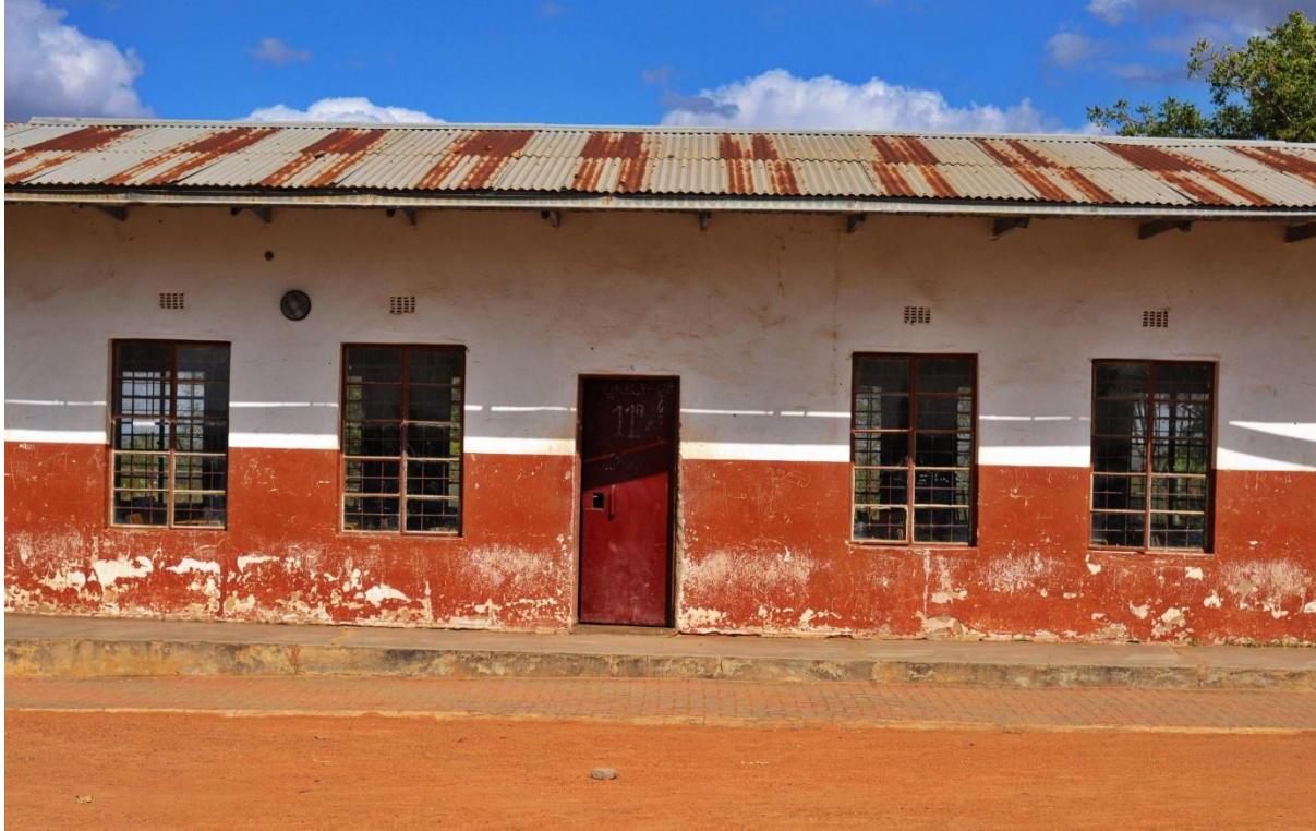
Fig 2. Netshimbupfe Secondary School. (Example of schools still found in South Africa. However, there are number of new ones built but still having huge backlog in some areas. This is Netshimbupfe Secondary School block built in 1975.) Photo by Lucas Ledwaba, 8 June 2020.
