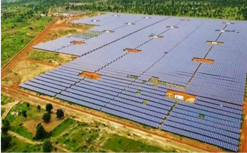
Figure 1 : Aerialview of the Zagtoui solar power plant.
