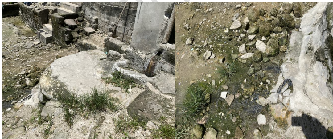
Figure 3: Leakage in a sanitation facility
