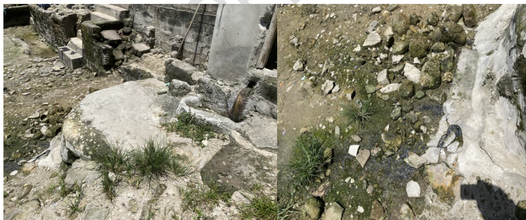
Figure 3: Leakage in a sanitation facility
