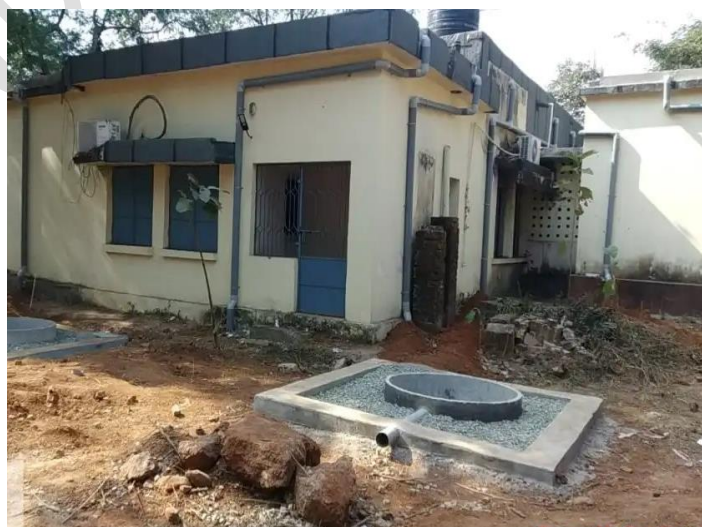
Fig 22: Rooftop rainwater harvesting in the Sukinda Block office
