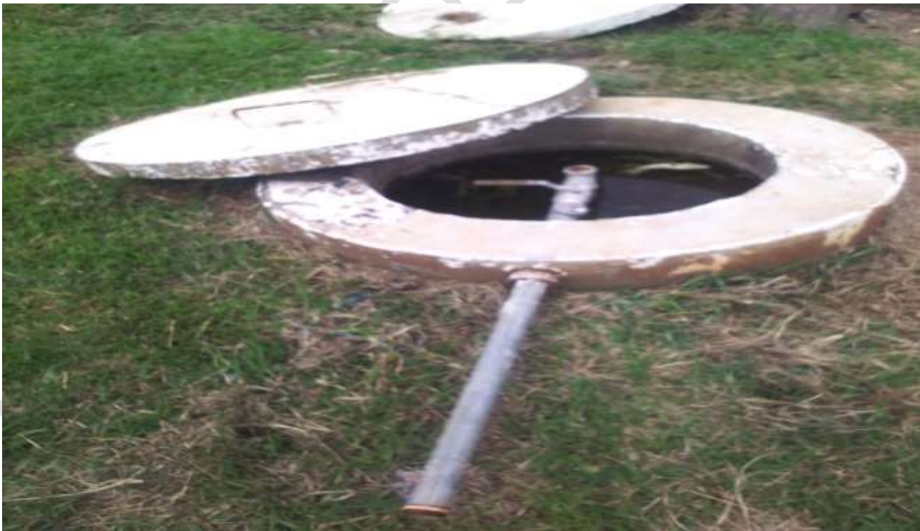
Figure 5. Example of a Fixed dome biogas plant as captured at Manchinchi Sewage Treatment Plant under Lusaka Water and Sanitation Company Limited.
