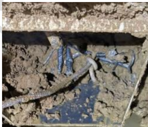
Fig. 8. difficulty in discharging slag
