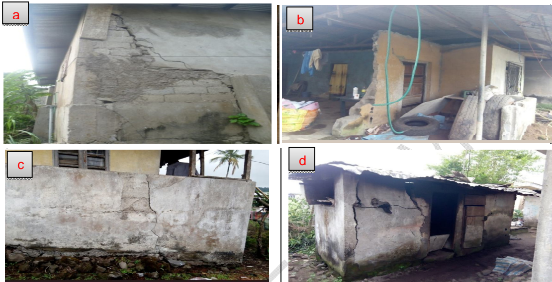
Fig.8. Damaged buildings in Buea during 1999 eruption (a & d Soppo, b. poto-poto quarter-Bogwango and c. Buea Town)
