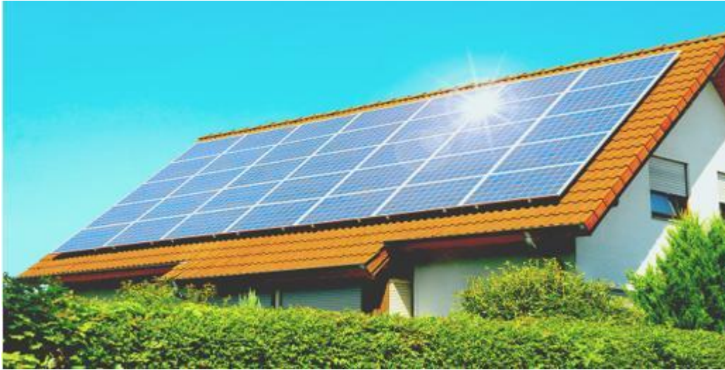
Figure 2: Roof-mounted Solar panels (source: Stern, Burke and Bruns, 2019)
