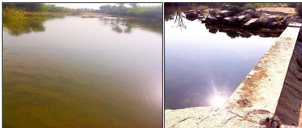
Fig 1: Small-scale irrigation facilities in the watershed
