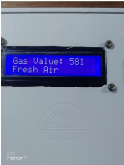
Fig. 10. Result screen of air quality monitoring system in ppm
