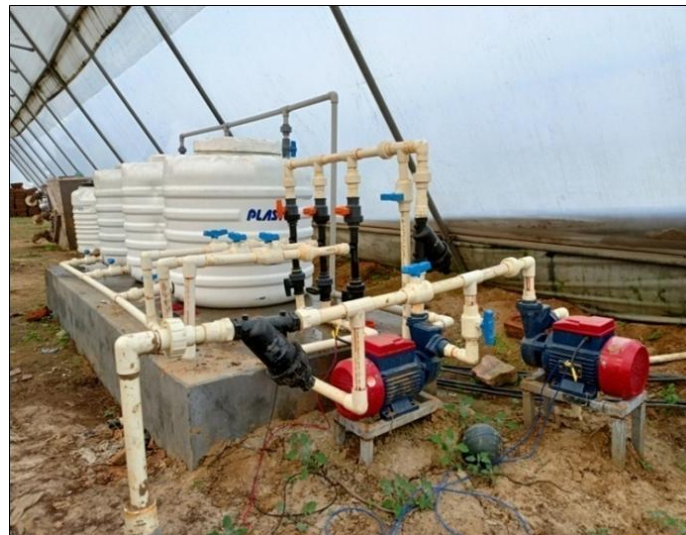
Fig. 6 Field view of developed fertigation control head
