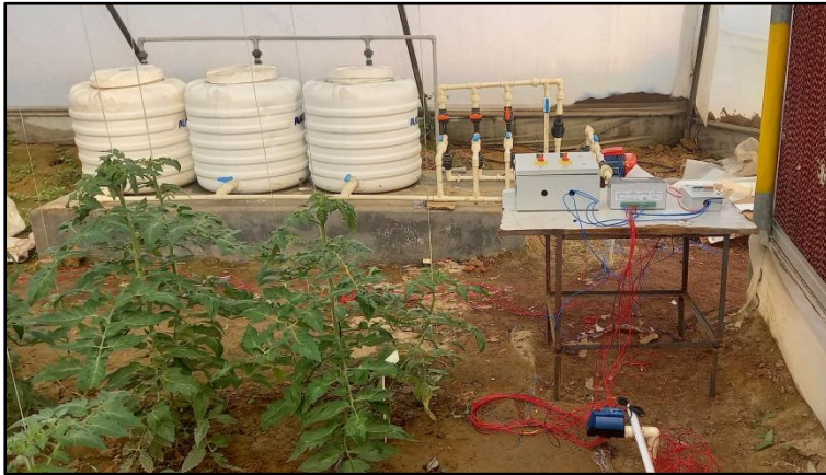
Fig. 17 Overall view of developed fertigation control head
