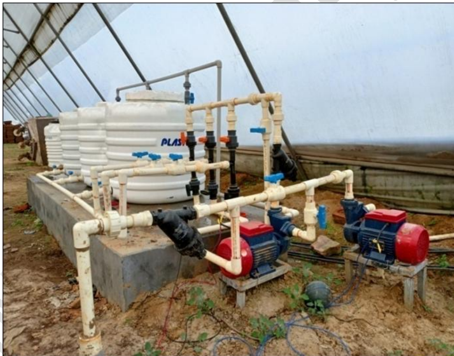
Fig. 6 Field view of developed fertigation control head
