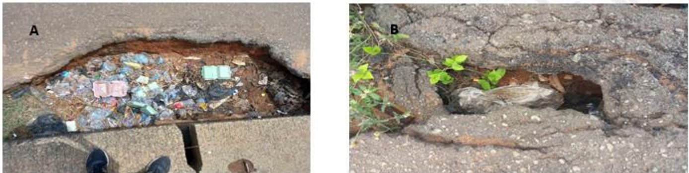
Figure 2. (a) Sinkhole at Awka site 1 (b) Soil pipe at Awka site 2
