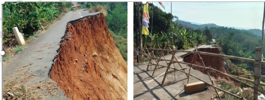
Fig 2. Landslide conditions in Bandungan hamlet, Kalongan Village
