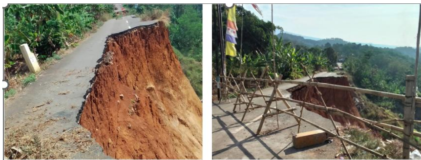
Fig 2. Landslide conditions in Bandungan hamlet, Kalongan Village
