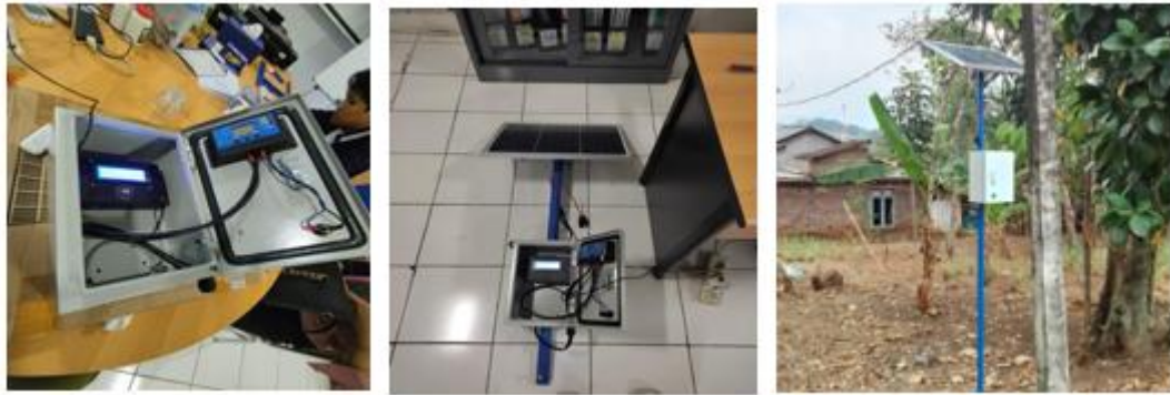
Fig. 4. Landslide Early Warning System
