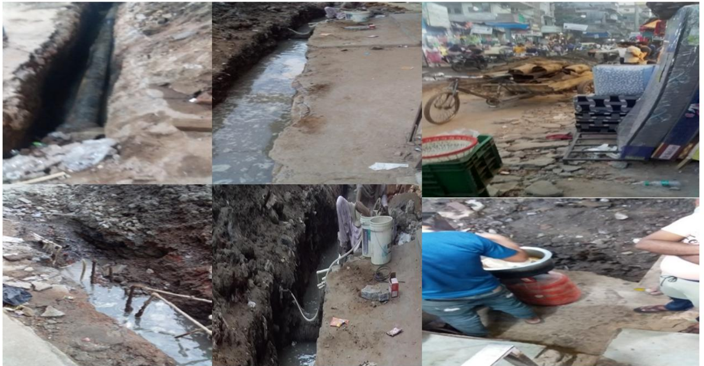
Figure 1 Pipeline repair pit and Scrapped rusted metal pipeline transported in cycle rickshaw without cover. Right bottom – food vendor near pit repair selling rotis that can lead to ingestion of soil dust
