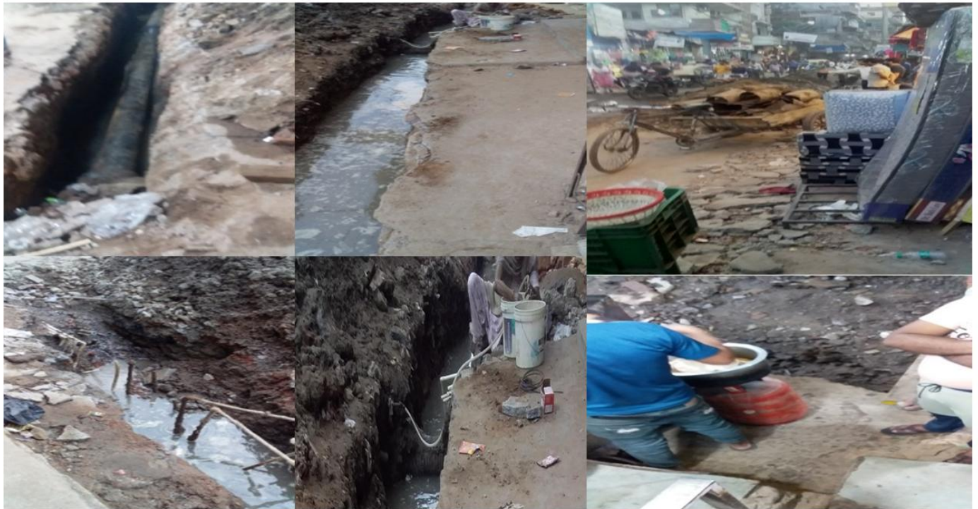
Figure 1 Pipeline repair pit and Scrapped rusted metal pipeline transported in cycle rickshaw without cover. Right bottom – food vendor near pit repair selling rotis that can lead to ingestion of soil dust
