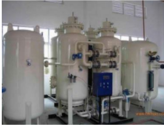
Fig 3: A Pressure swing adsorption (PSA) Unit in a Hospital
